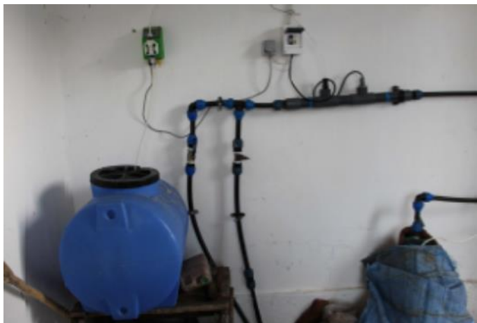
Figure 4-6: Sodium hypochlorite dosing station, Negresti village
