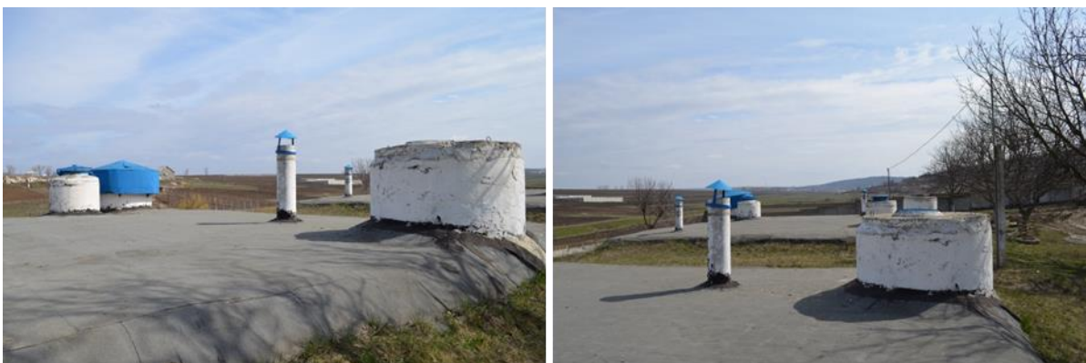
Figure 4-4: Water intake in Micauti village– underground water reservoirs with a volume of 500 m 3 each
