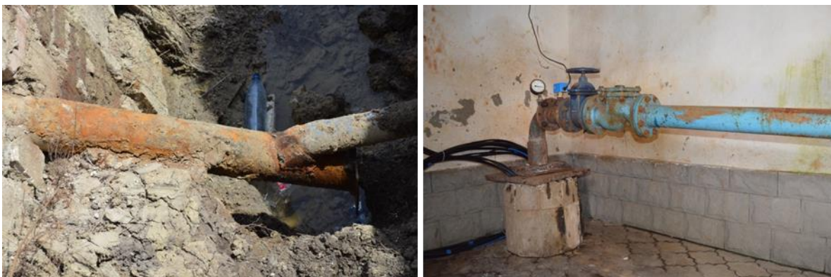
Figure 4-3: Water intake in Micauti village– deep well no.1 (3941) and pressure pipe to underground water reservoirs
