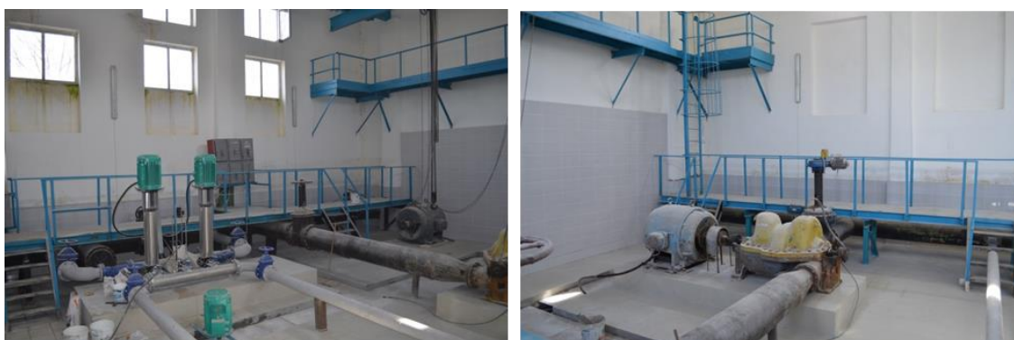
Figure 4-7: Second level pumping station (PS-2): set of pumps WILO Type Helix V 5209-2-3/25/E/K/400-50 and reserve pump ЦHC 400/210
