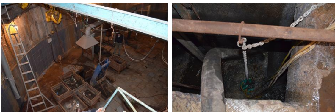
Figure 4-15: Main wastewater pumping station
