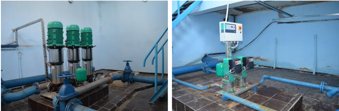
Figure 4-8: Third level pumping station (PS-3)
