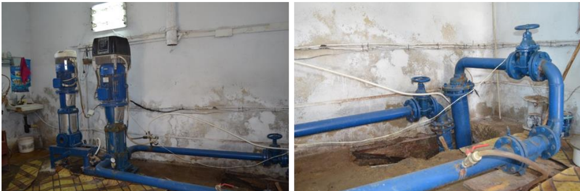
Figure 4-9: Third level pumping station (PS-4)
