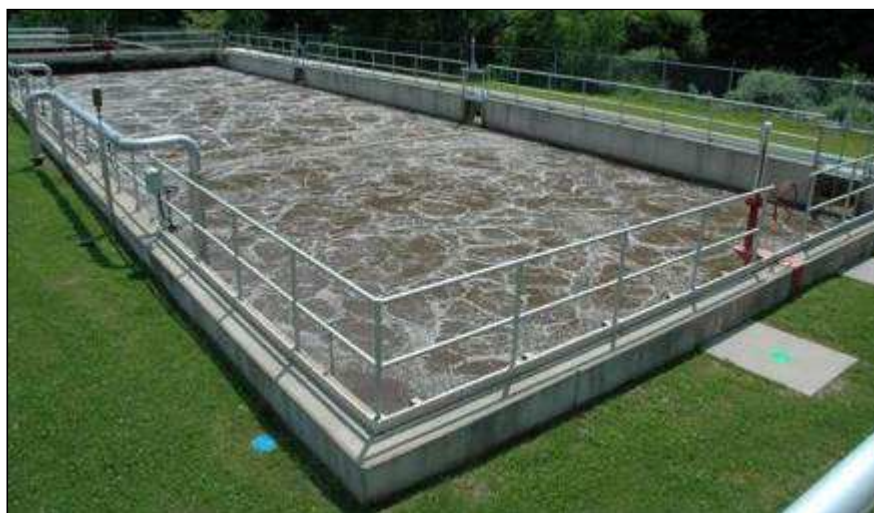
Figure 9-4: Activated sludge aeration tank, Source of image: T. Simmons/Indiana University of Pennsylvania
